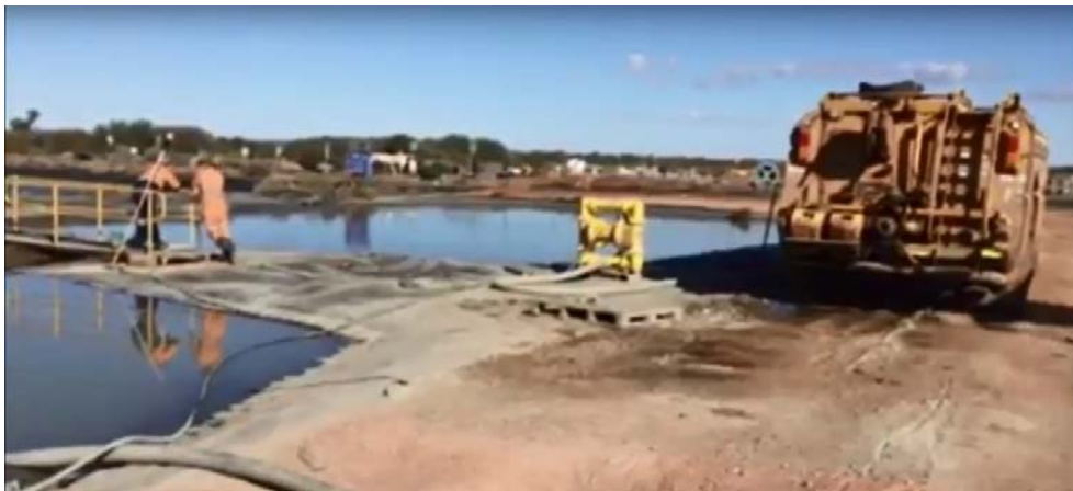
Mine Dewatering Pump
